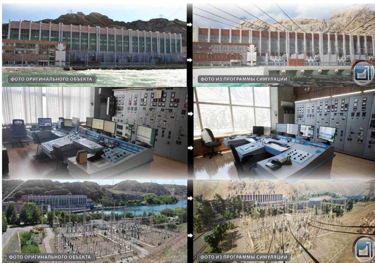
Figure 3 – Comparison of the Main Control Console: Actual HPP Control Panel (left) and Virtual Interface in the Simulator (right)
